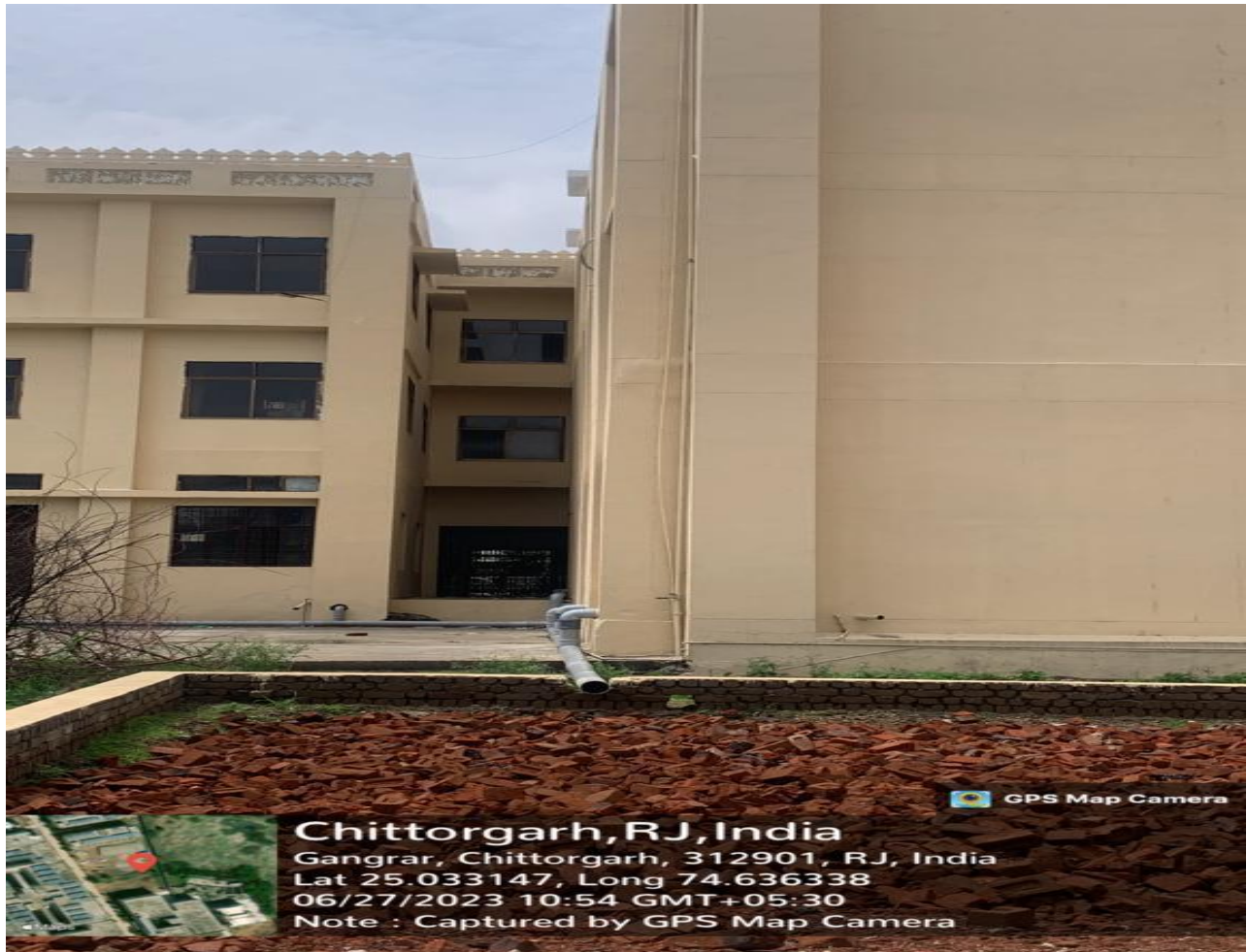
Rain Water Harvesting
